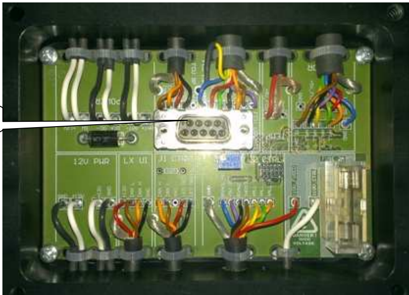
FCC (FES connecting circuit) box opened
